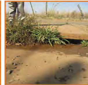
Picture 5: Sunken and partially blocked kerb inlet
