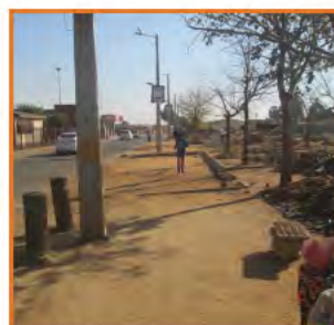
Picture 15: Section of missing paving
