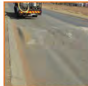
Picture 7: Mechanical damage on speed hump
