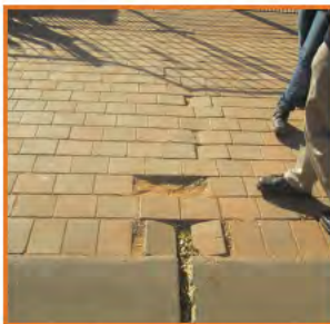
Picture 11: Poorly reinstated paving
