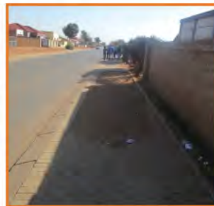
Picture 12: Missing paving
