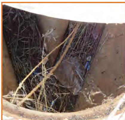
Picture 2: Debris in the dry unused manholes
