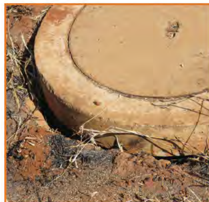
Picture 3: Manholes starting to deteriorate
