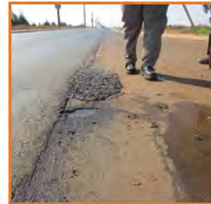
Picture 4: Poor patch repair and pothole
