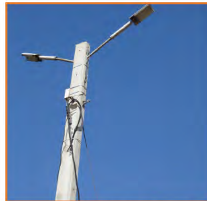
Picture 16: Vandalised wiring
